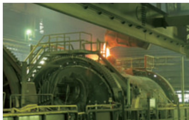
Anode furnace at Saganoseki Smelter & Refinery
