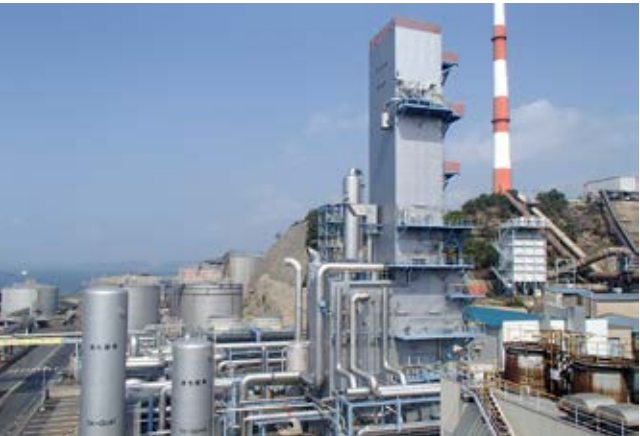
Oxygen production system at Tamano Smelter, Hibi Kyodo Smelting
