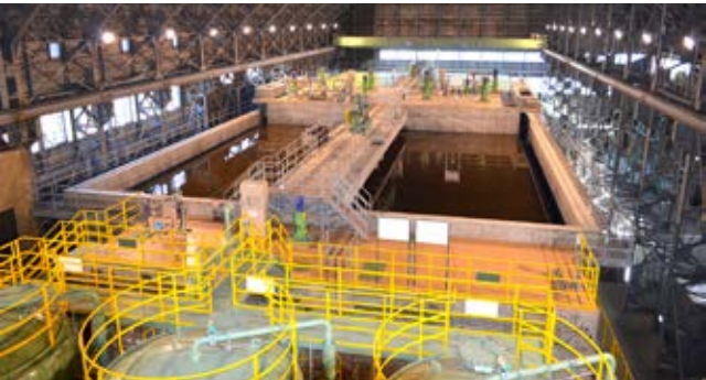
Motoyama AMD treatment facility at Toyoha Mine
