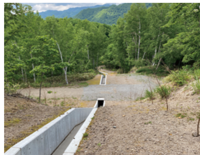
The drainage canal of the Toyoha Mine Ishiyama tailings dam, completed in FY2022
